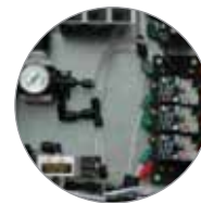
Pneumatic control systems
