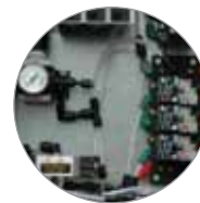
Pneumatic control systems
